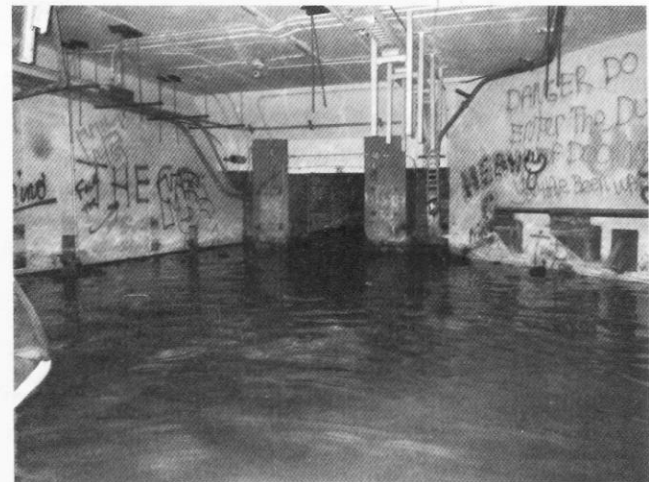
Inside the second blast lock. The blast door leading to Launcher Area 2 is in the centre of shot while that for Launcher Area 3 is out of shot to the right.
